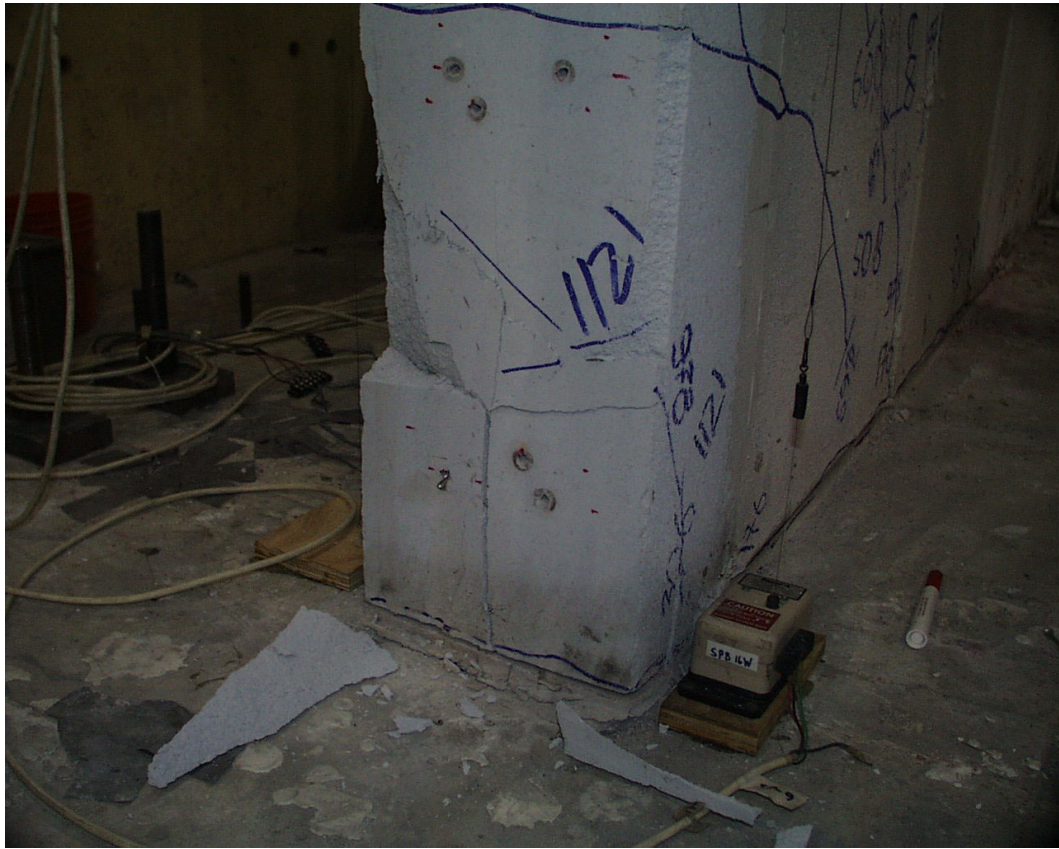
Figure 3.9: Spalling at the north end of Shear Wall Specimen 17
