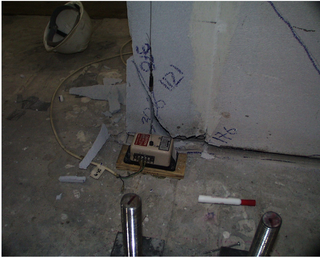
Figure 3.10: Toe crushing north at north end of Shear Wall Specimen 17
